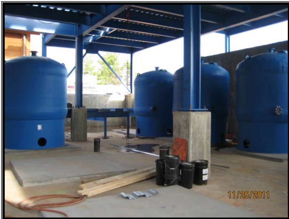
Back of House FRP Tanks
