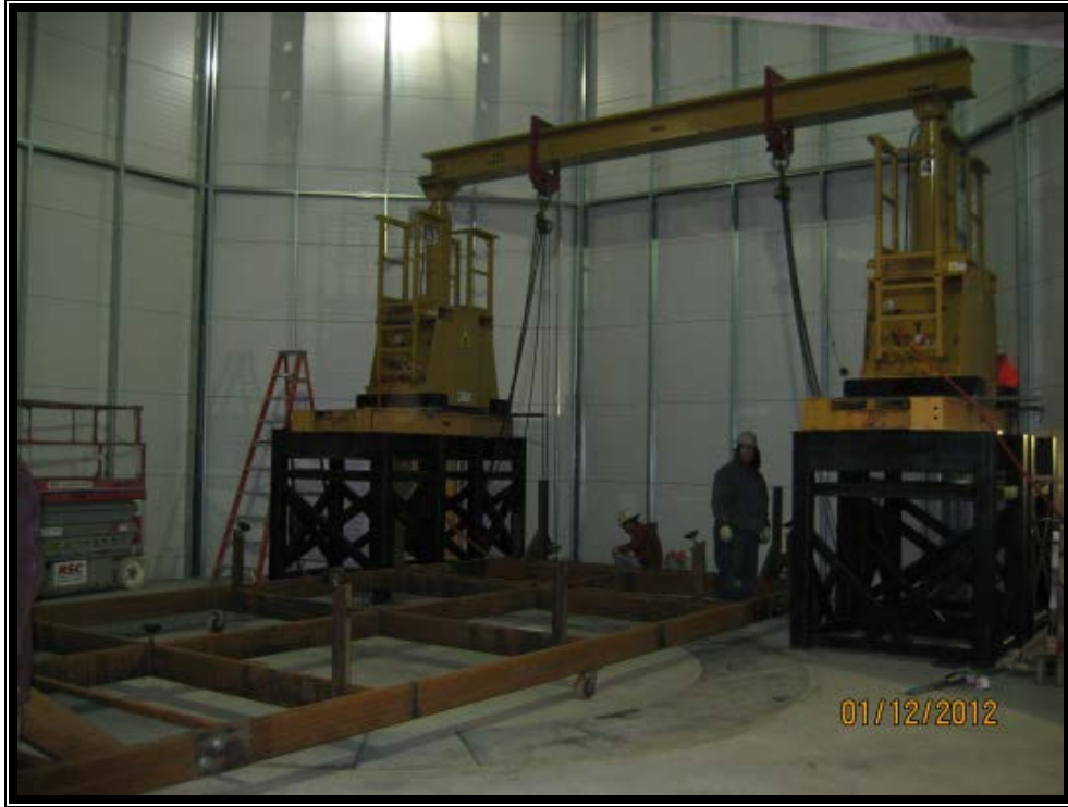
Stingray Tank Gantry Crane
