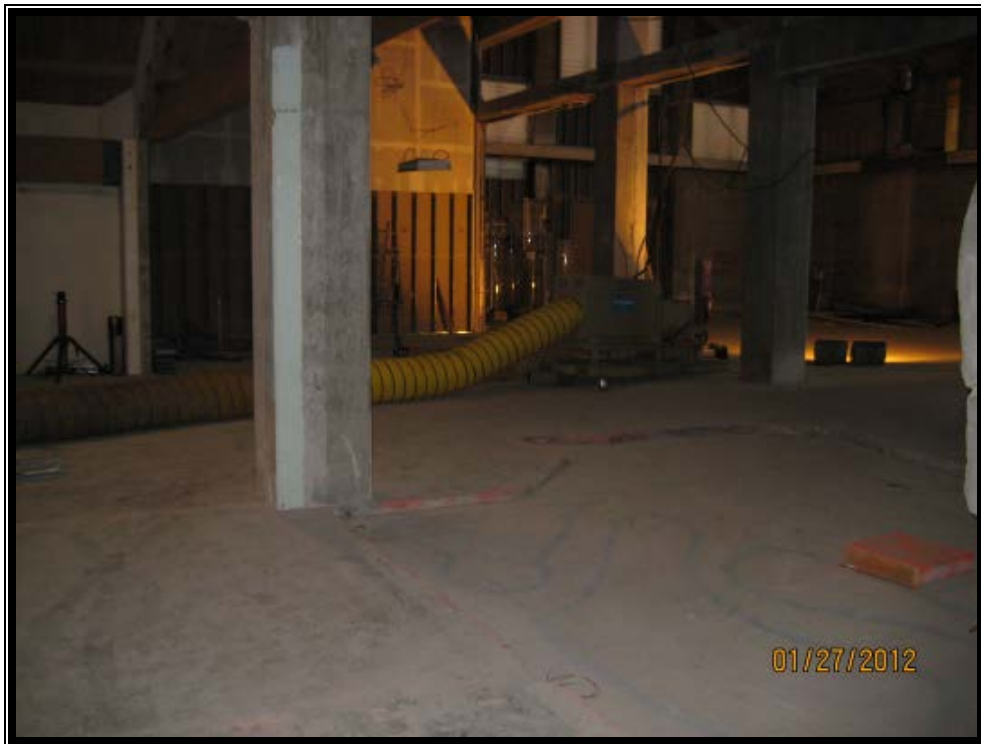
Second Floor Temporary Heat
