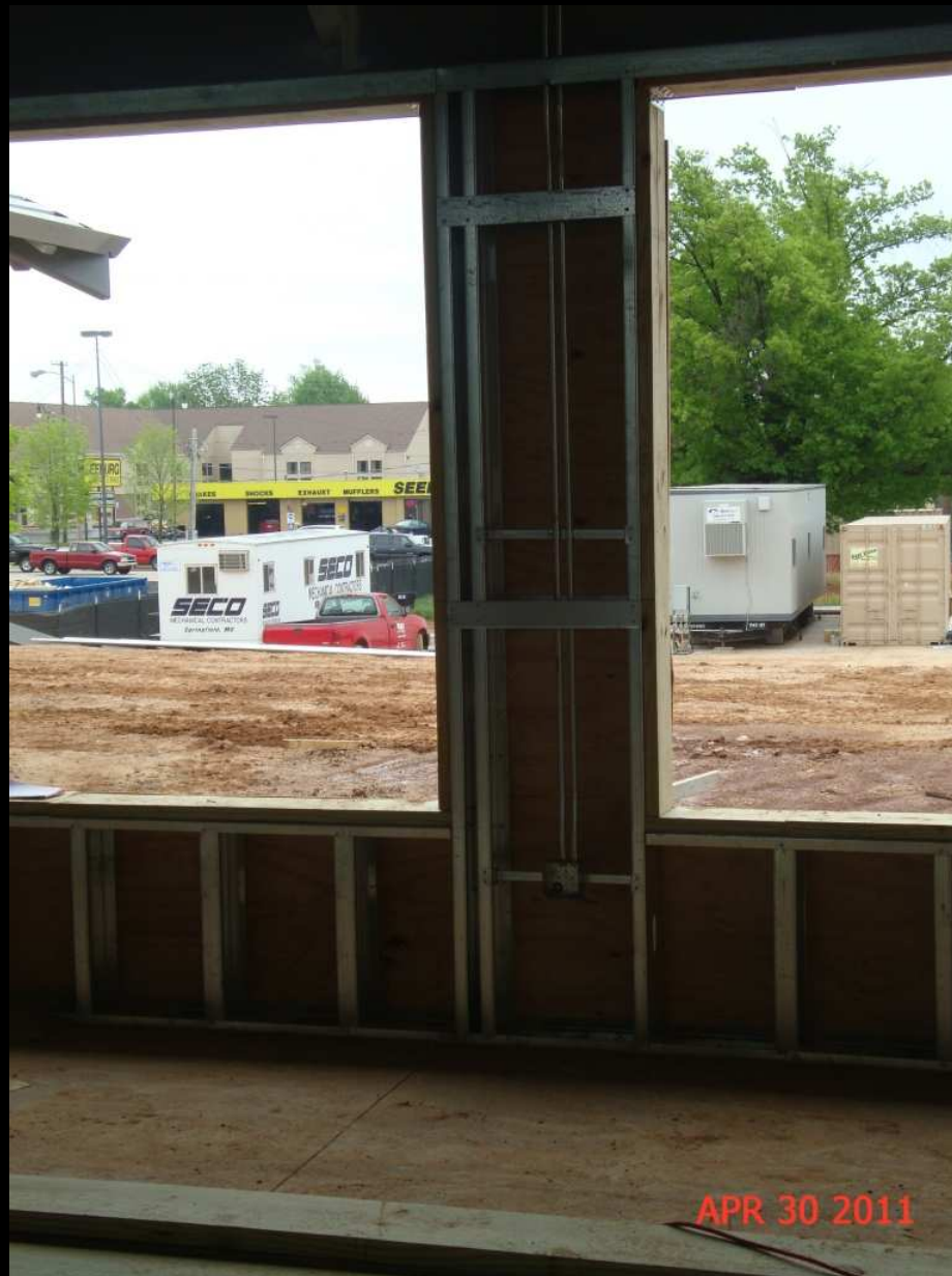
Electric In Wall
