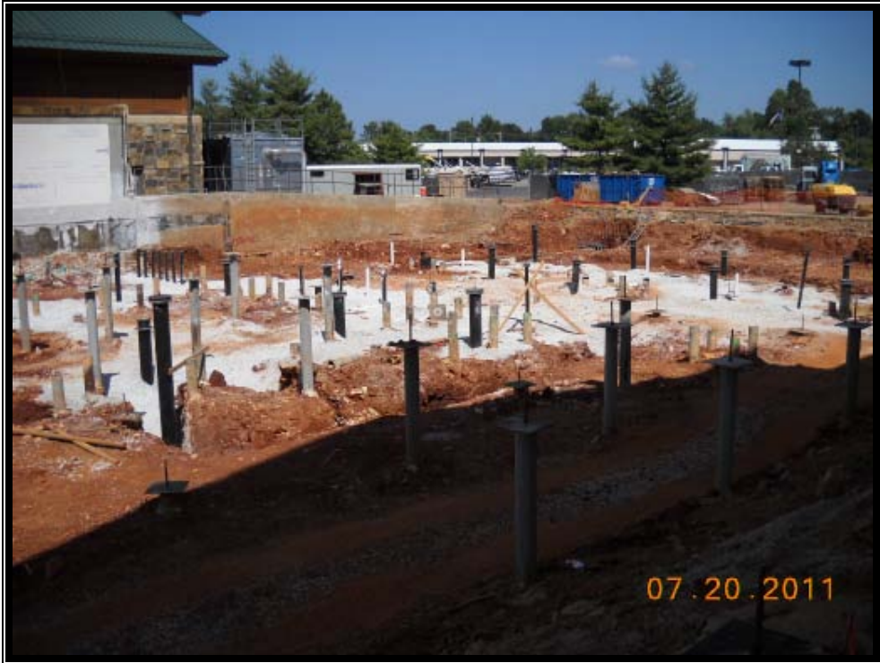
Back of House LSS Pipe
